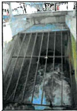
Undersized Culvert Inlet
